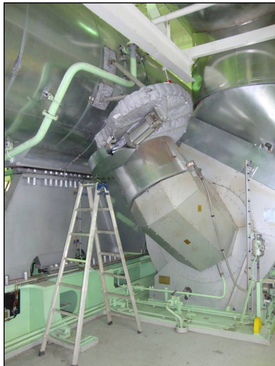
Figure 5. 12K98ME main engine on Maersk Salalah. An insulated swing gate valve for turbocharger cut-out installed between the exhaust gas receiver and the turbine side on one of the three turbochargers.
